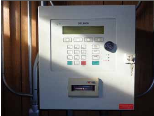
19. View of the AST monitoring system.
