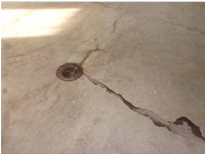
23. View of staining within the automotive garage.
