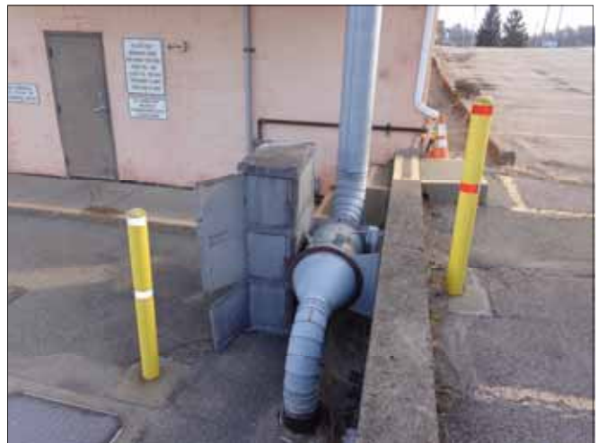
10. View of the ventilation system for the AST vault.
