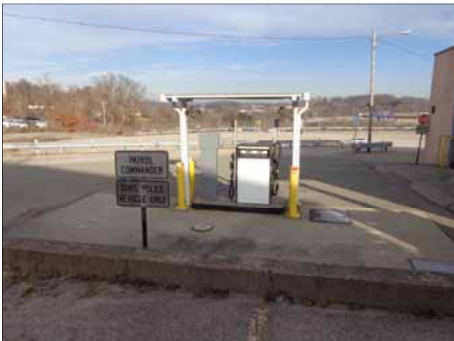
5. View of the 10,000 gallon AST and Pump.
