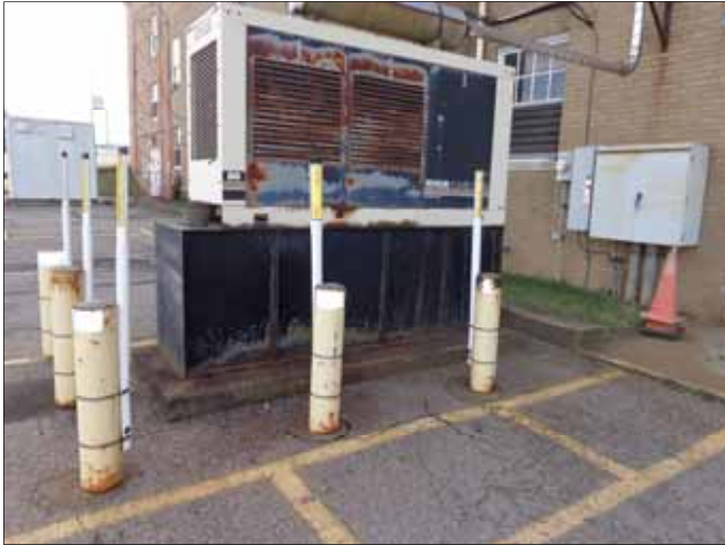
13. View of an onsite diesel generator.
