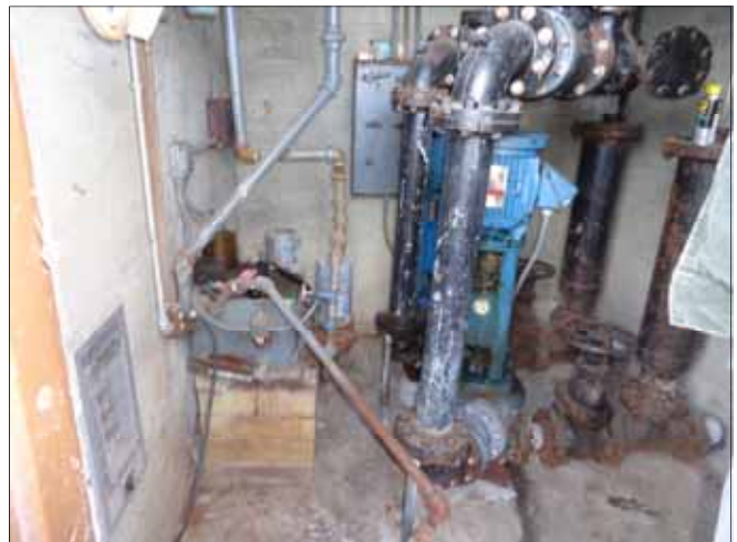
24. View of the sanitary pump system.
